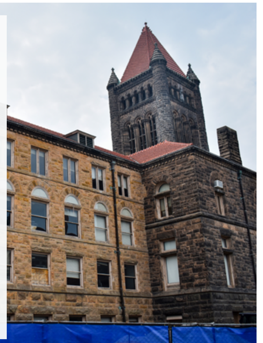
Cleaning crews have been working throughout the summer to restore the exterior of Altgeld Hall. This east side view of the building shows the contrast between cleaned and untreated stone. | Photo credit: Shelby Koehne
